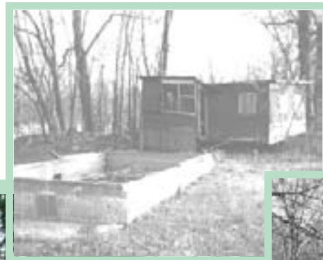
Structures damaged by the flood of 1982 in Fenton.
